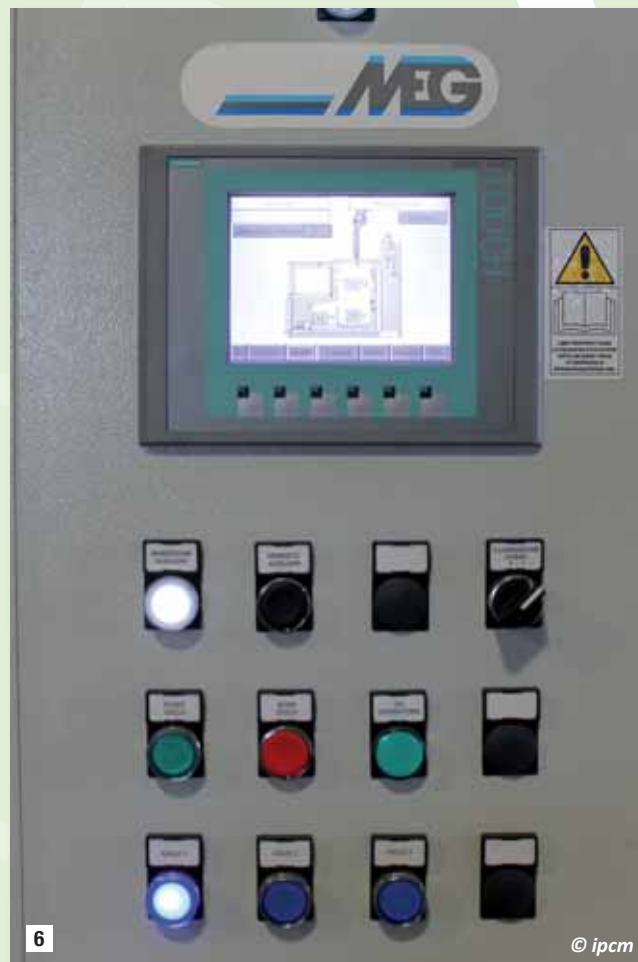
6 The control panel of the new solvent-based cleaning plant.
