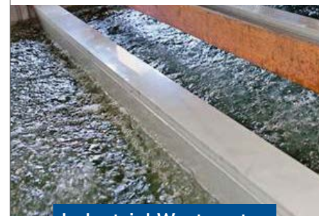
Industrial Wastewater Treatment
